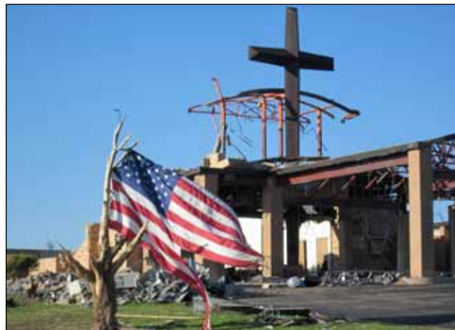
Pictured above is an unnamed church in Joplin after it was struck by the May 22 tornado.
